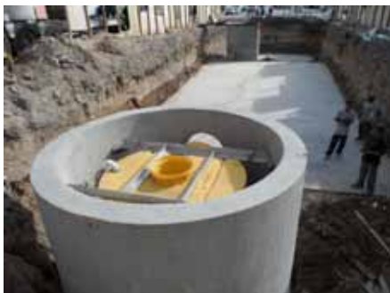
Fig.2 An 8-ft Downstream Defender® (pictured above) and a 6-module Up-Flo® Filter were used to treat harvested stormwater.
