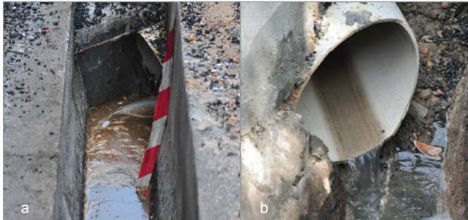
Fig.4(a) Pre-installation and (b) post-installation effluent in a storm trench where the 4-ft diameter Downstream Defender® was installed.
