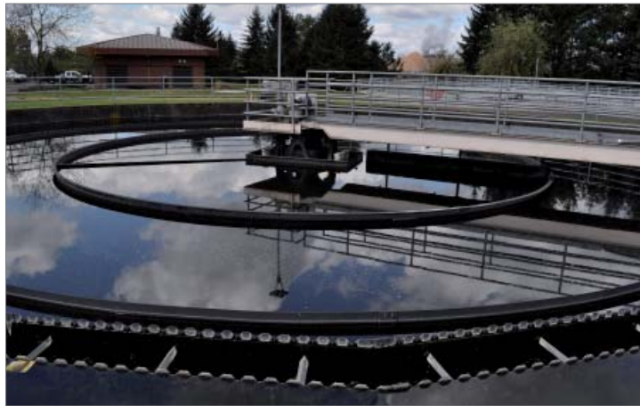
Primary Clarification System
