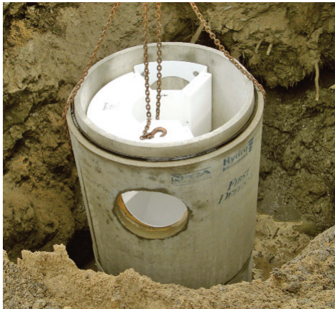
Fig. 2 “Maintenance of the vortex separator is easy. Periodic cleaning once or twice a year with a vac truck to remove debris is required.” Says Penza.
