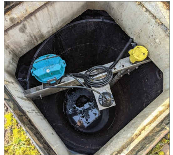
The Hydro-Logic® Smart Monitoring system installed in the Downstream Defender®
