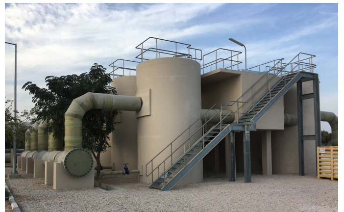
The project incorporated an unconventional above-ground installation
