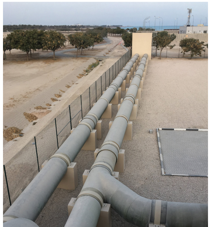
The treatment facility pumps stormwater for treatment before discharge into the Arabian Gulf
