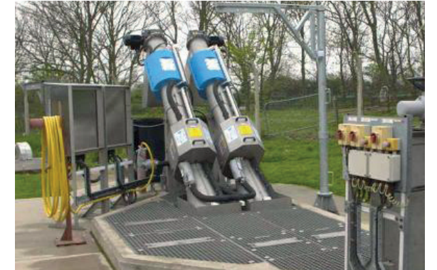
Packaged inlet works
