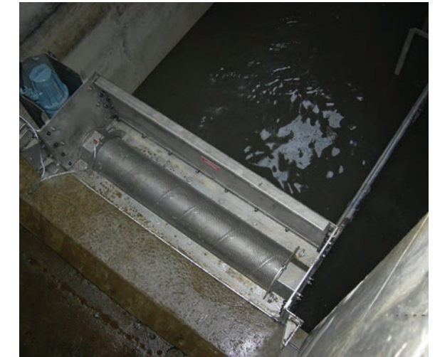
Powered, hydraulically cleaned screening
