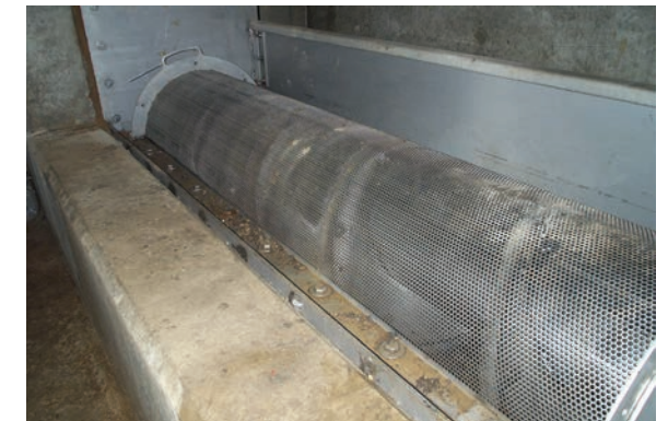
Storm tank pre-screening
