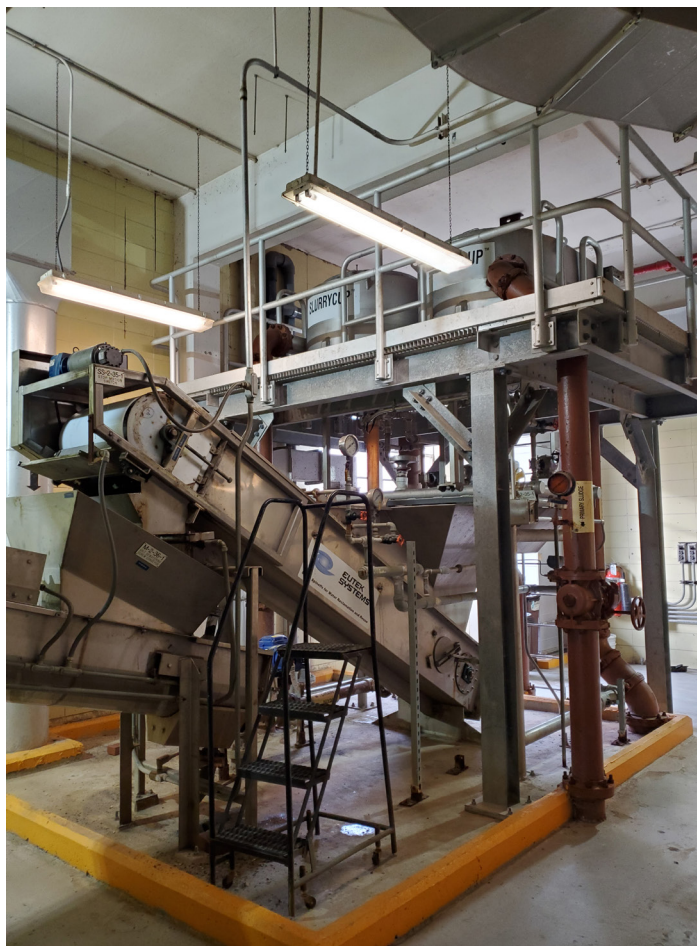
Clavey Road's Sludge Dewatering SlurryCup / Grit Snail System in 2021
