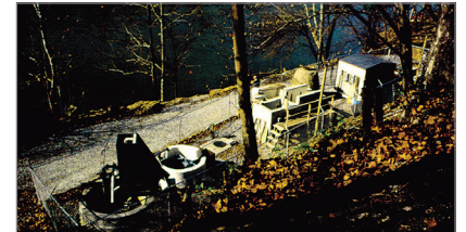
Piloting on the banks of the Chattahoochee River helped Columbus evaluate Hydro International’s vortex separator as an alternative to conventional options
