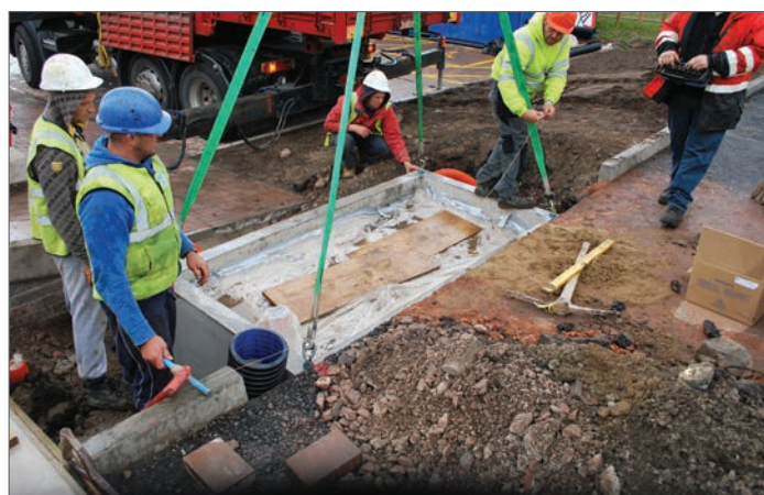
Chamber showing protective fabric and boards covering the filter media.
