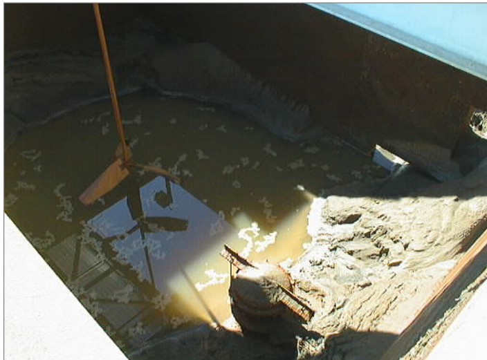
Conventional Flocculation Tank
