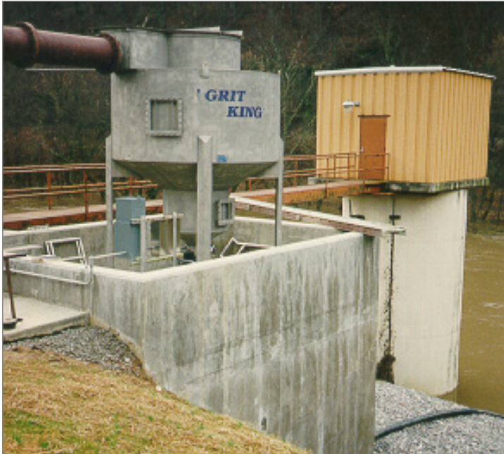
Prestonburg, KY WTP influent pre-treatment with Grit King®
