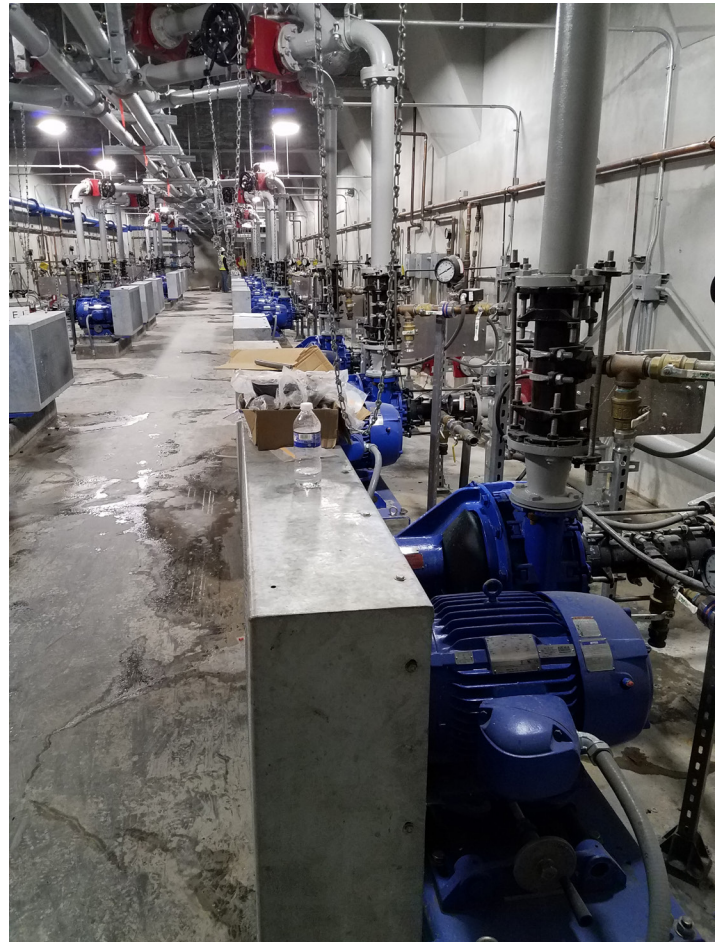
Grit Underflow from HeadCell Systems at RM Clayton Plant
