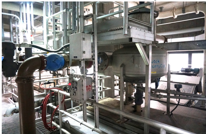
Operating SlurryCup / Grit Snail System 16 Years After Installation
