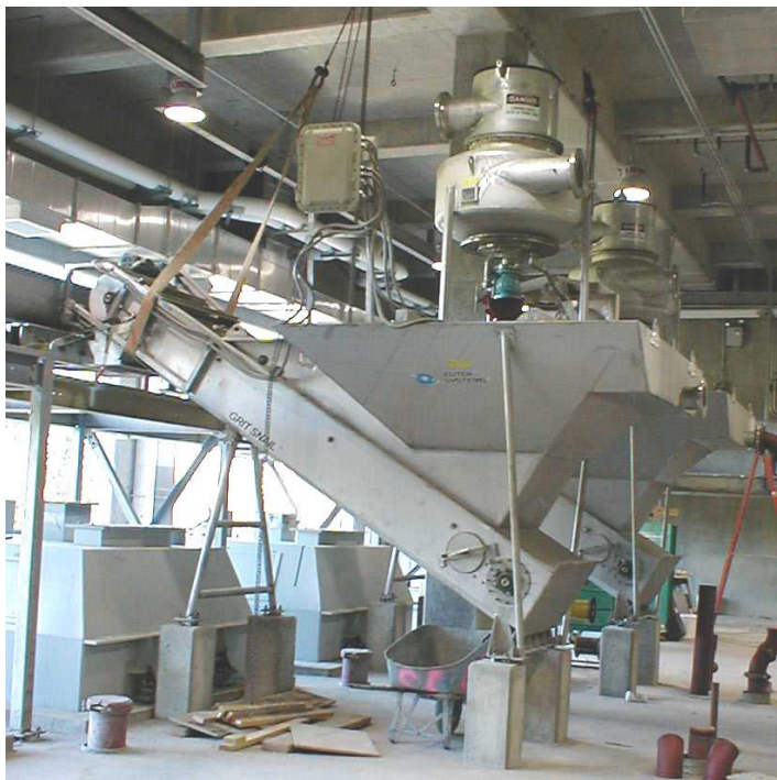
Rock Creek's System During 2002 Installation
