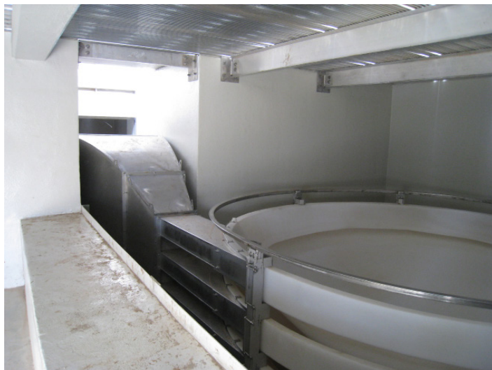
One of Tupelo Bayou's installed HeadCell® grit separation systems
