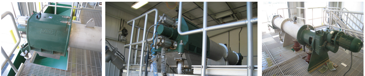
Conway Arkansas's Hydro-Sludge® Screen system allows the WWTP to land apply their treated sludge
