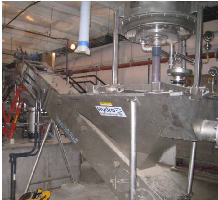
One of Tupelo Bayou's installed Grit Snail® grit dewatering systems
